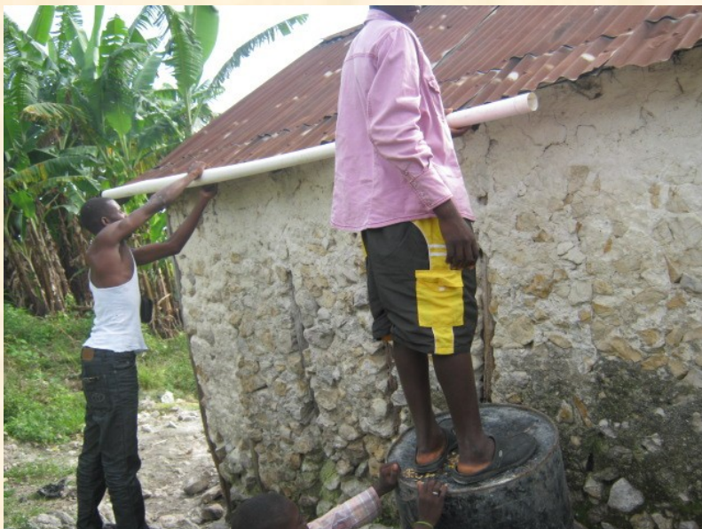
Installing rain-water collection systems in the mountain community. So far 12 have been installed, and we hope to install 30 in the near future.
